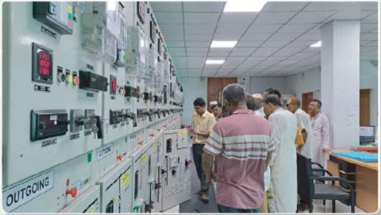
Practical training at Central Sub-Station, Khulna.
