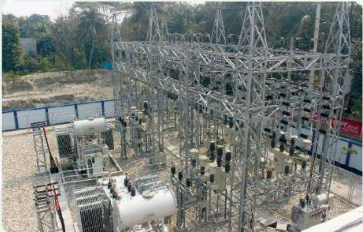
Newly Constructed 33/11 KV 2x10/13.33 MVA Substation, Fultola, Khulna.
